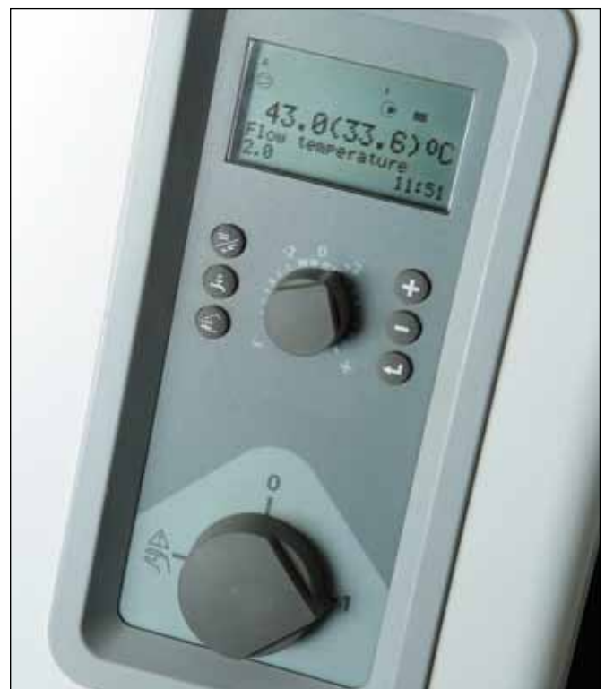
Installers must work with customers to ensure that they understand how to use the controls
