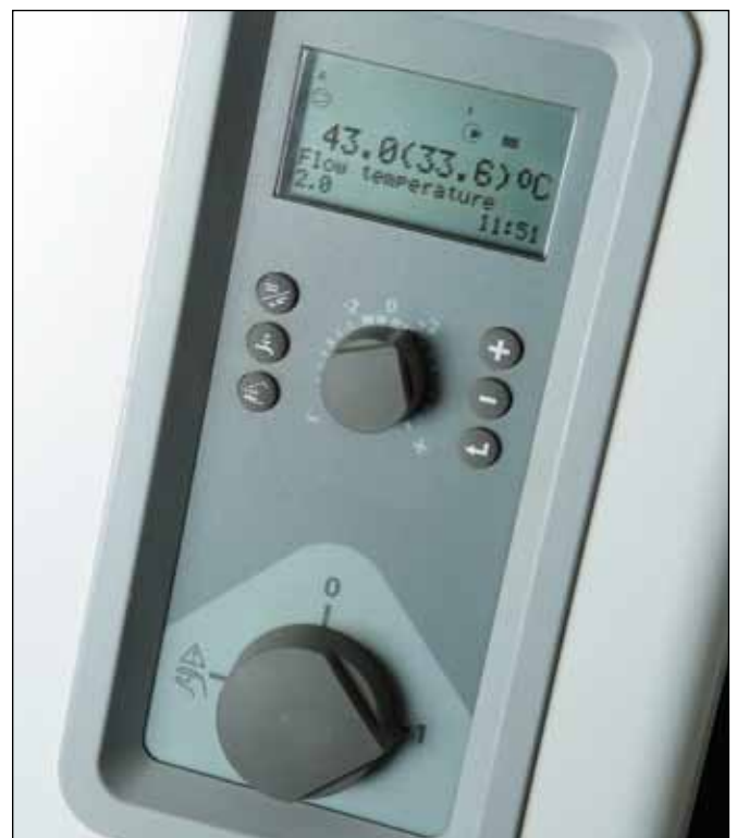
Installers must work with customers to ensure that they understand how to use the controls
