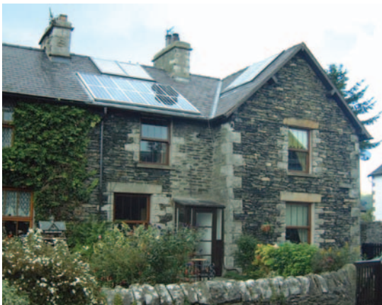
Figure 7 PV array and solar water heating collectors installed on a house in Cumbria
