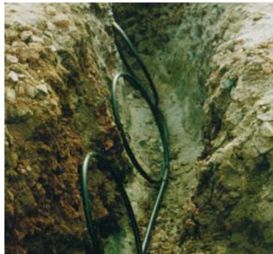
Ground loop collector for a GSHP © Geoscience 2002
