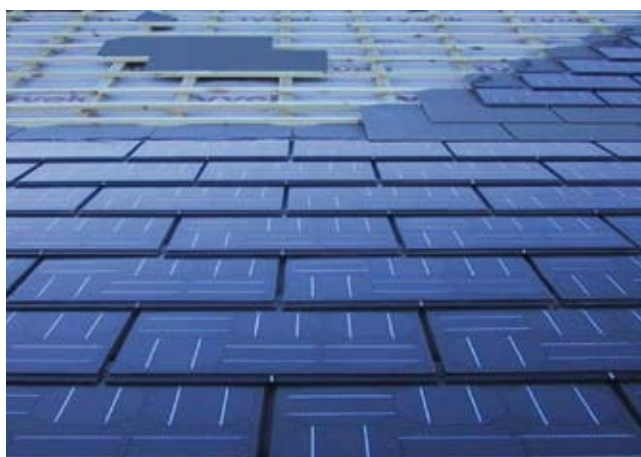
A domestic PV array
